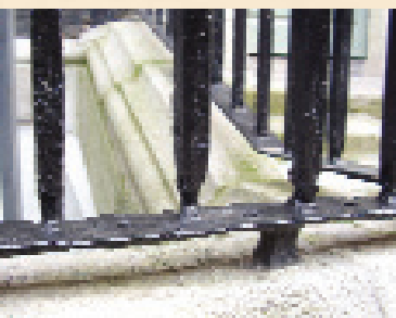
Above Top: Unless done by an appropriately skilled blacksmith, repairs and replacement of wrought iron sections are likely to be unsuitable and not in keeping with the character of the original ironwork
