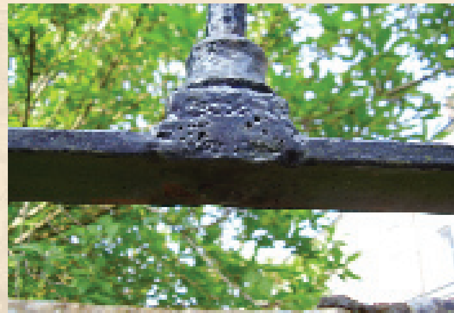
Below: Paint cannot fill holes. Casting flaws such as those pictured above should be filled to prevent water becoming trapped and causing corrosion to develop.
