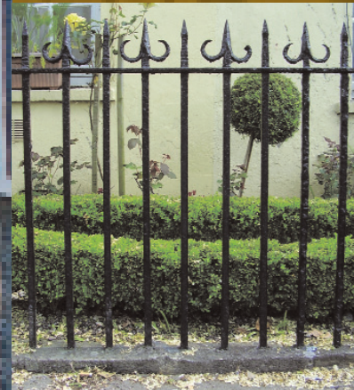
Above: Typical Georgian railings on Dyke Parade where the bars run directly into the plinth and plain finials alternate with scrolled finials; a decorative central panel enlivens the streetscape
