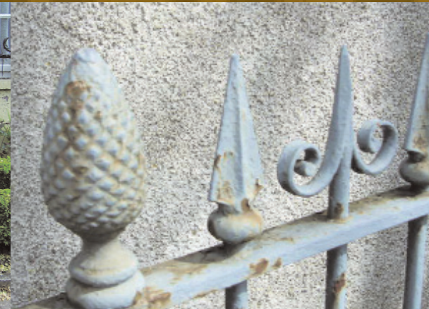
Above: In Ashton College, Old Blackrock Road, three types of finial are used with the cast iron pine cones articulating the corners and the stouter bars
