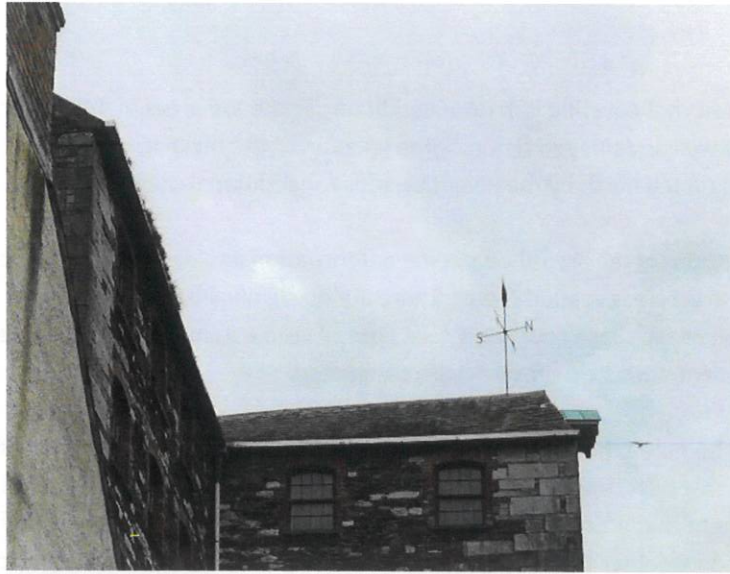
Fig.14 Gutters and downpipes
